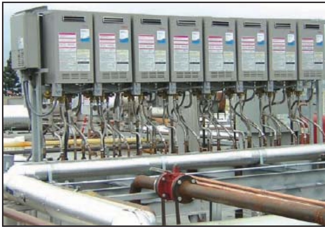
The installation consists of 28 WaiWela tankless water heaters plumbed in parallel on two fabricated, galvanized steel skids on the roof of the plant.
